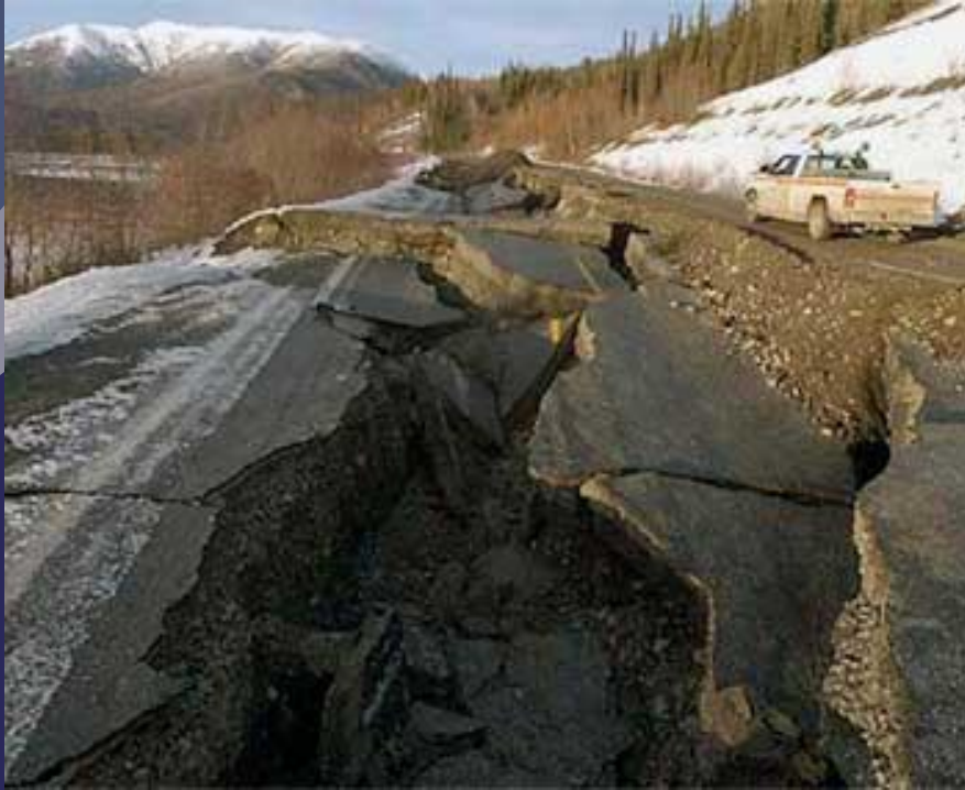
This rupture of the Tok Cutoff Highway in Alaska resulted from a magnitude 7.9 earthquake along the Denali Fault in 2002.
