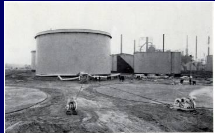
An 8-ton winch for pulling and a 4-ton winch for side restraint were used for moving this 250-ton tank on the Stanlow, Cheshire, Refinery of Shell U.K. Ltd.
