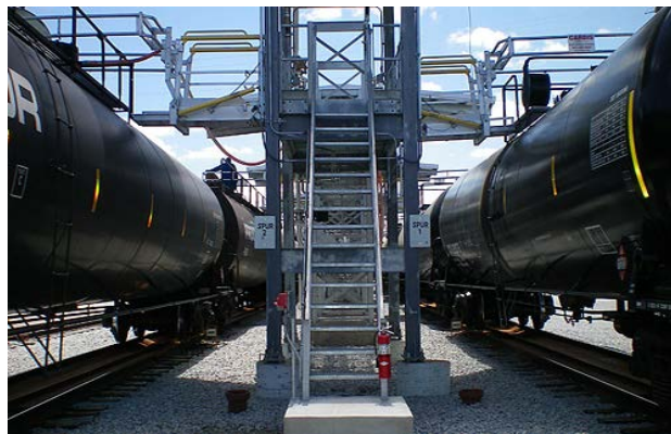
Figure 12 Paired Loadout Tracks
